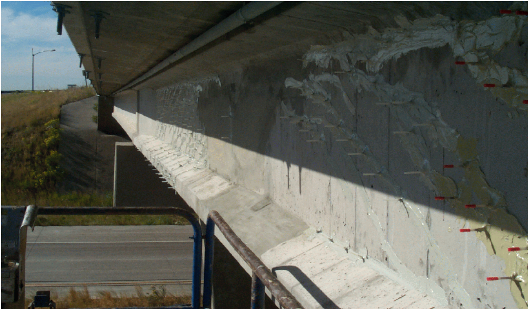
Fig. 3 - The Damaged Girder with Injection Ports in place
