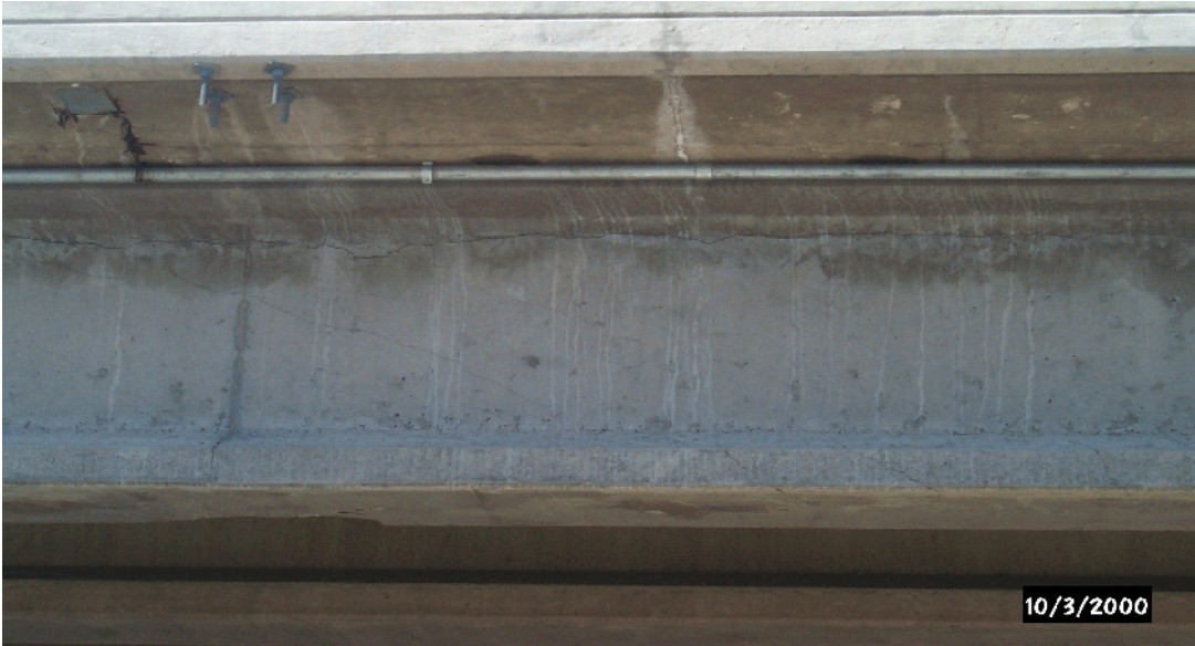
Fig. 2 - The Damaged Girder Prior to Epoxy Injection Repairs
