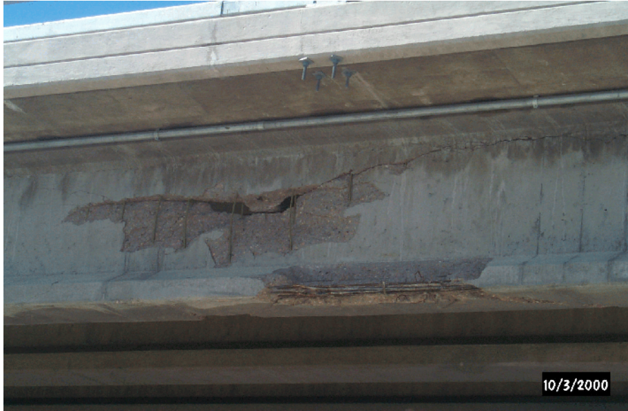
Fig. 1 - Damage on the Eastmost Concrete Girder before the Repairs
