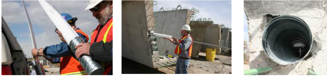
FIGURE 3 – STYROFOAM SUPPORTED BY WIRE ROD (LEFT), THE FOAM ROD BEING INSERTED INTO THE DUCT TO FORM VOIDS (CENTER) AND VIEW OF STYROFOAM DEFECT INSIDE A DUCT (RIGHT)
