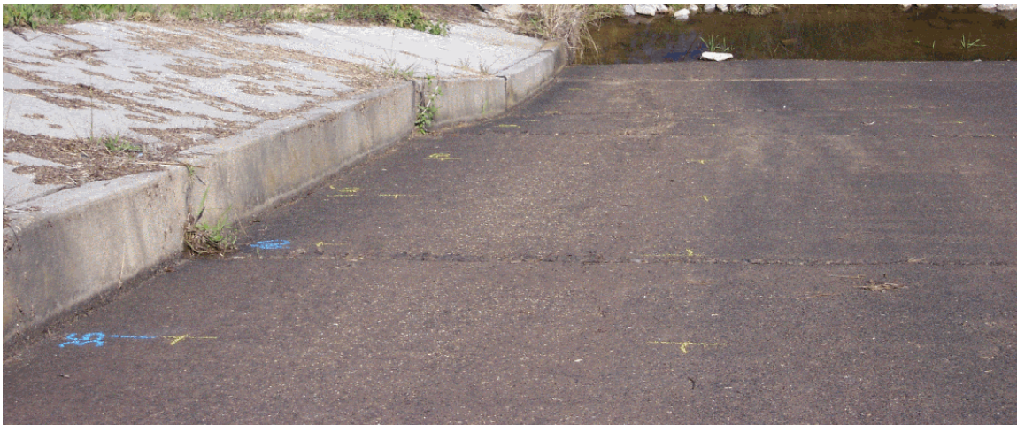
Fig. 6. Spillway Slab Showing Distortion of Concrete
