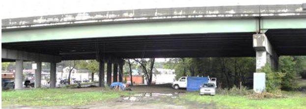
Figure 5. New Jersey Route 23 Bridge looking west – IBIS tested Girder 2W3 is in the background
