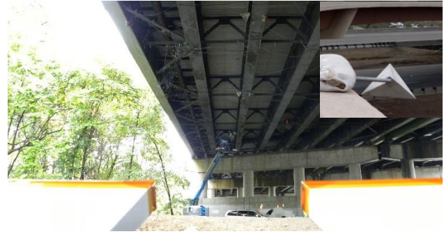
Figure 6. View over IBIS air horn antennas of the corner reflectors (see inset photo) at potentiometer locations on Girder 2W3
